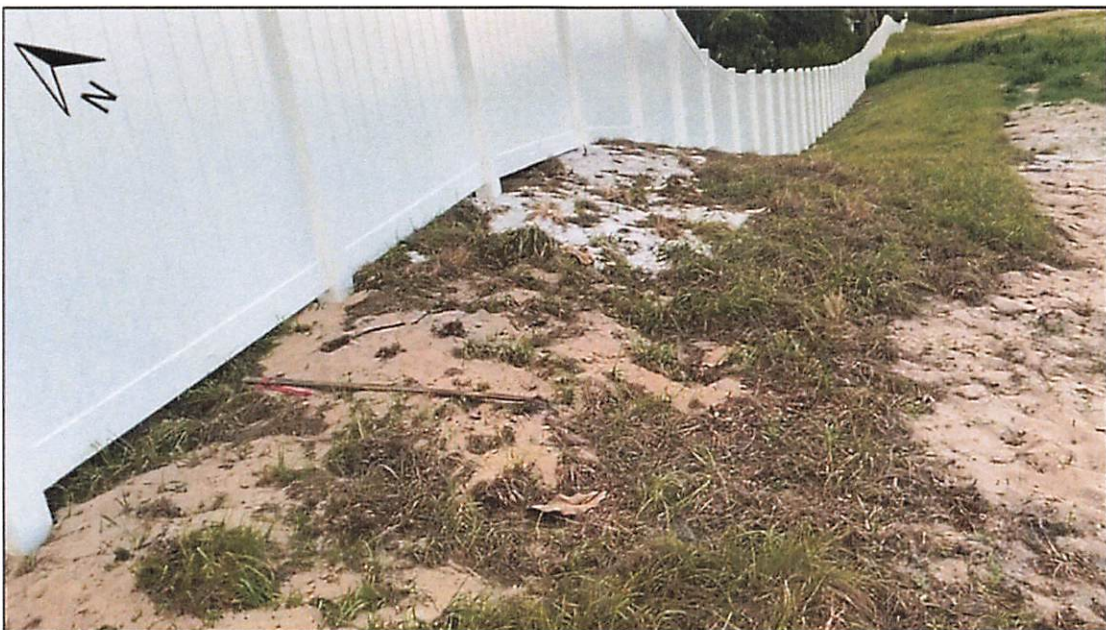
Seawalk on Dune Facing East: Sand Observed, possibly from digging fence posts
