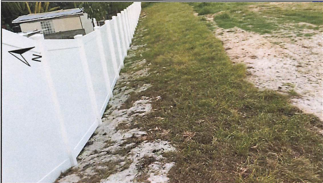
Seawalk Facing East: Sand Observed, possibly from digging fence posts
